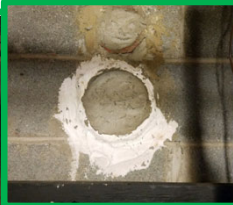
Capped emissions vent
