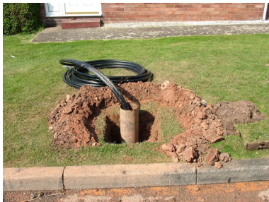
(B) Vertical Drilled Borehole
