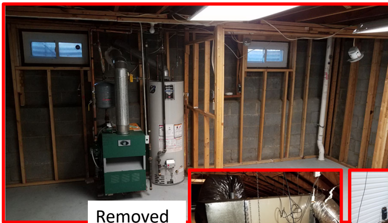
Before (natural gas furnace and hot water heater)
