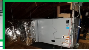
Attic air handler
